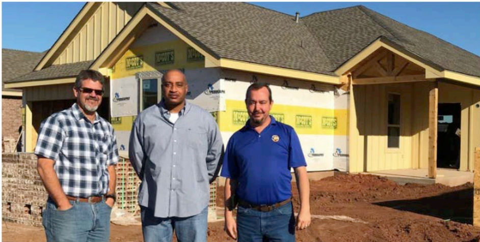
United States Air Force Chief Master Sergeant John A. Hammonds (center) visits a jobsite with Van Watson (left), assistant building official, city of Abilene; and Tim Littlejohn (right), building official, city of Abilene, during a ride-along that is part of the Code Council's new ICC Military Families Building Career Path Program.
