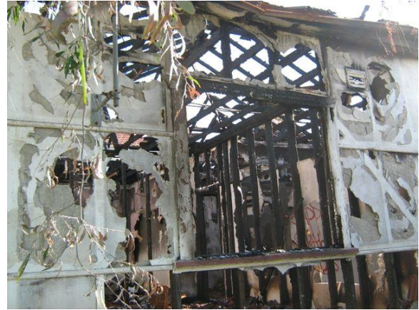
Asbestos in fire-damaged building
